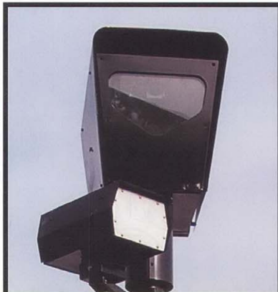
Enclosure was painted black as requested by the City of Chicago
